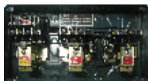
Interior View of MK1 SASD
