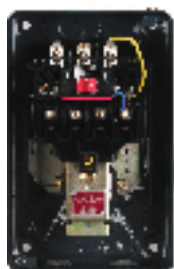
Interior View of MK1 DOL
